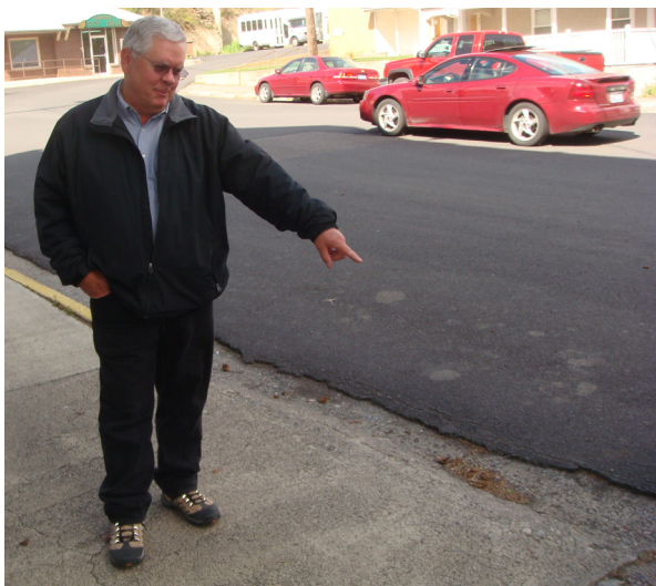
Mayor Alan Gould points to the loading area at the Senior Center with its deteriorated sidewalk and gutter, which flood from rain and snow.
